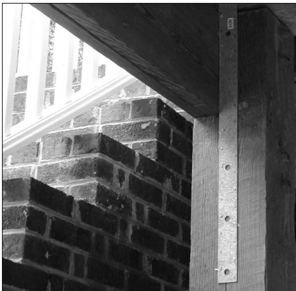
The hurricane straps seen here are an example of how a structure can be reinforced to survive severe winds.
